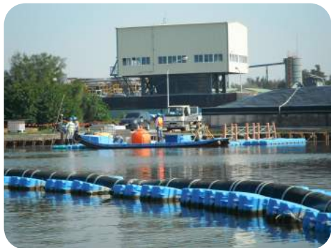
Pipeline on the pond
