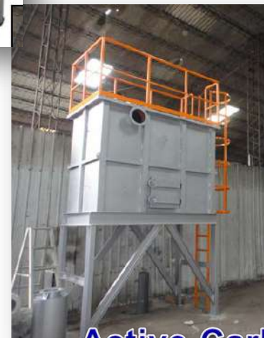
Active Carbon Tank
