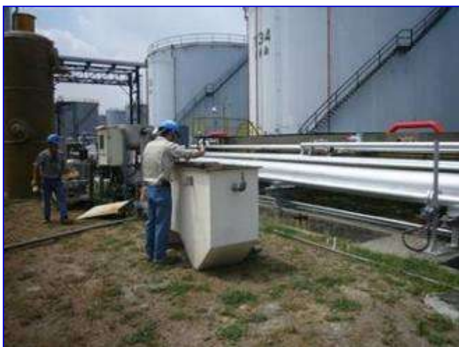
Oil & Water Separator
