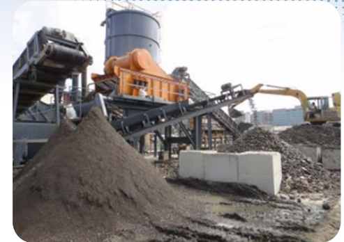
Washed soil discharge
