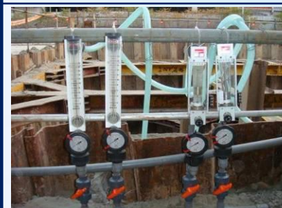
3. Flow meter and control valve
