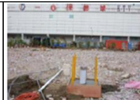
5 newly-installed monitoring wells
