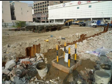
3 newly-installed monitoring wells
