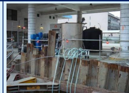
2. Injection tank and pipe
