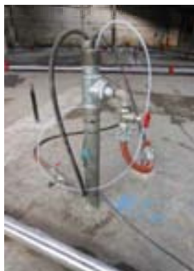
DUAL PHASE RECOVERY WELL: water abstraction via bottom-loading pneumatic pump and vapour extraction via connection to side channel blowers
