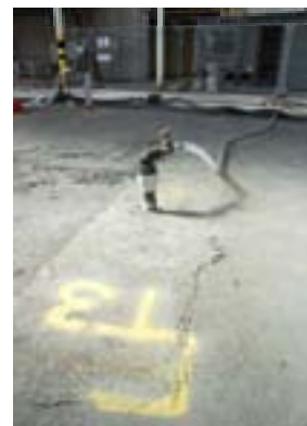
TRENCH AND TRENCH RISER WITH CONNECTION TO RECOVERY SYSTEM
