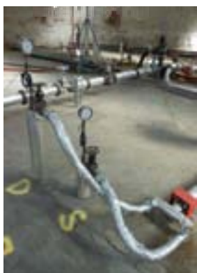
SHALLOW AND DEEP STEAM INJECTION WELLS WITH PRESSURE GAUGES
